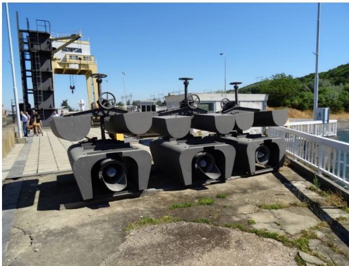
Figure 3.13 - Navigational lock "Djerdap I", devices for creating water vortexes
