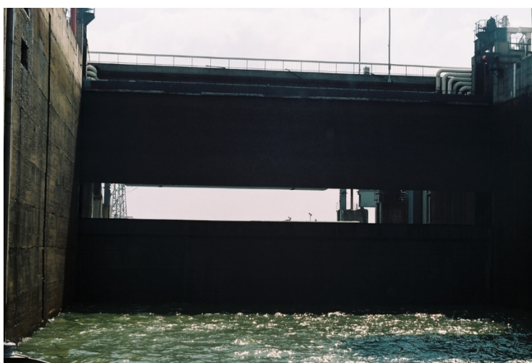
Figure 3.9 - Navigational lock "Djerdap I", middle head, main double door
